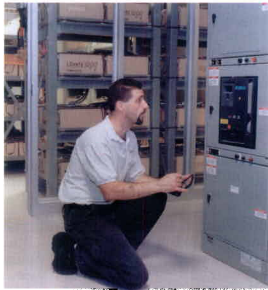
A UNICCO technician conducts an inspection of UPS backup equipment. The data can be entered on the spot and then uploaded into Maximo for processing.
